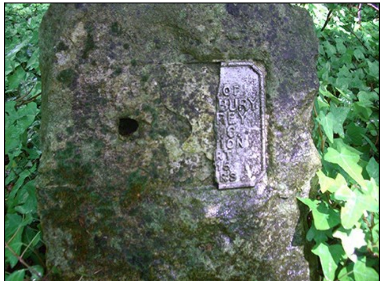
War Memorial 2 has a damaged plaque which is half missing © Angela van der Horst, 2014
