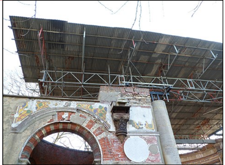
War Memorial 1 is unstable and there is significant damage to the materials © WMT, 2012
